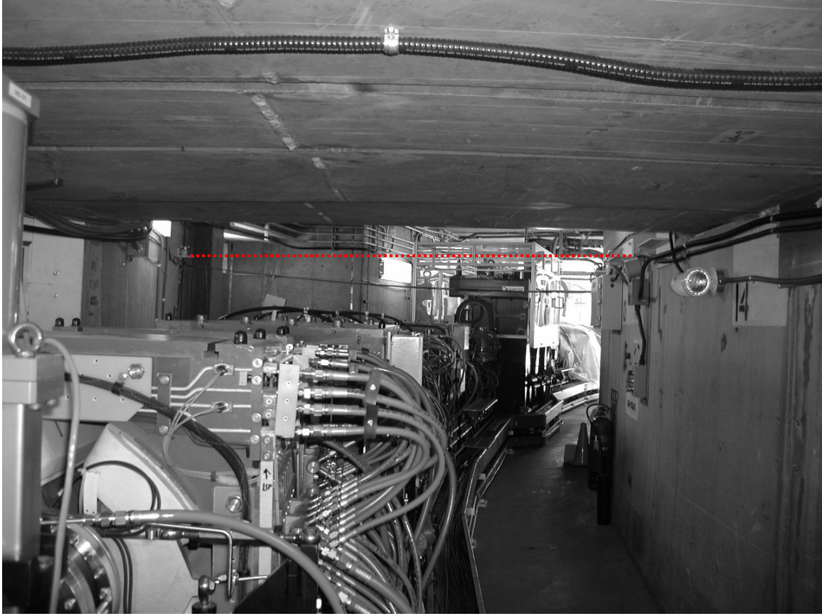
Figure 4 Laser beam path wall to wall
